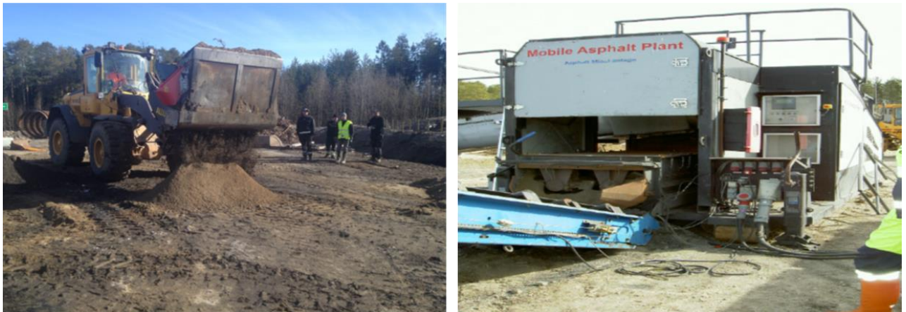
Figure 5: A construction loader and asphalt plant used in mixing till and GLDs (Mäkitalo et al., 2015).
