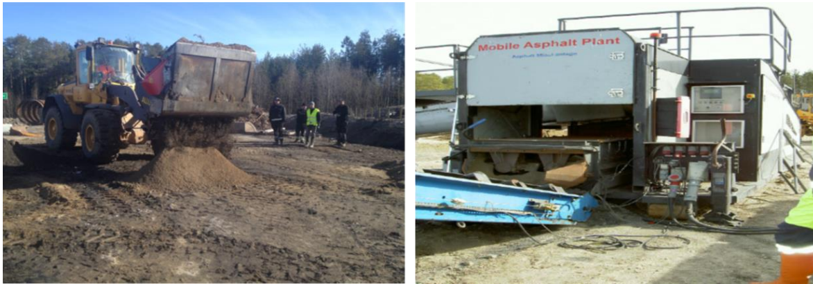
Figure 10: A construction loader and asphalt plant used in mixing till and GLDs [7]
