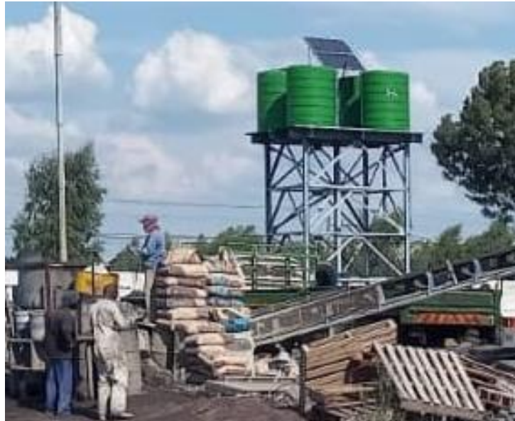
Fig Figure 2: Water storage
