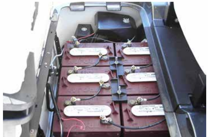
Deep cycle batteries
