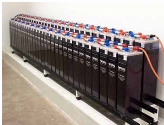
Reserve batteries or battery bank
