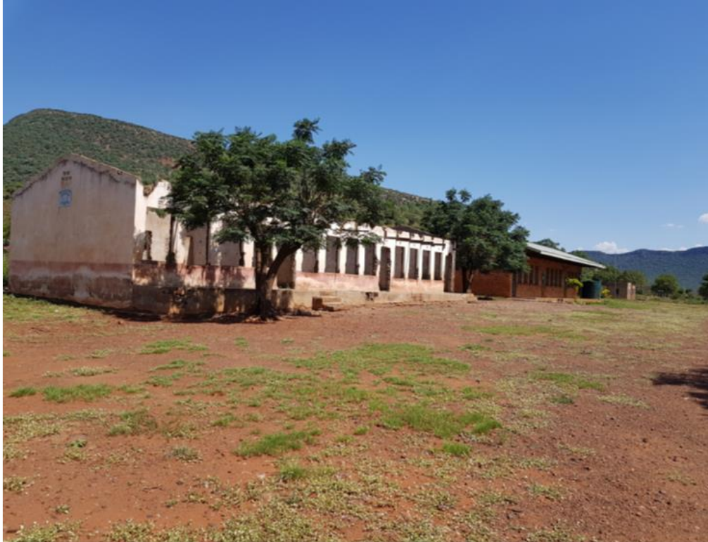
Before: Classrooms made of asbestos material
