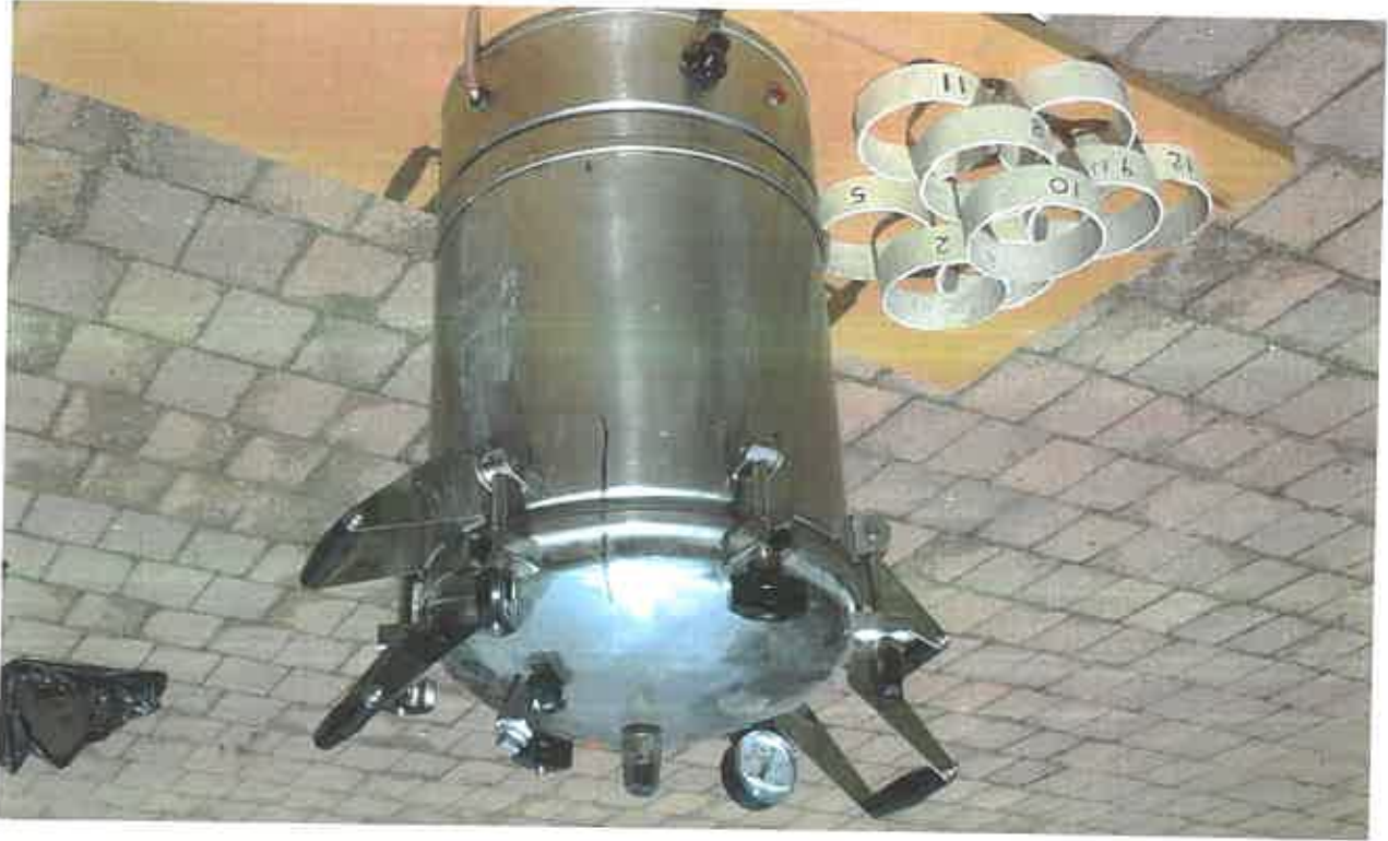
Figure 12: Low pressure steam vessel
